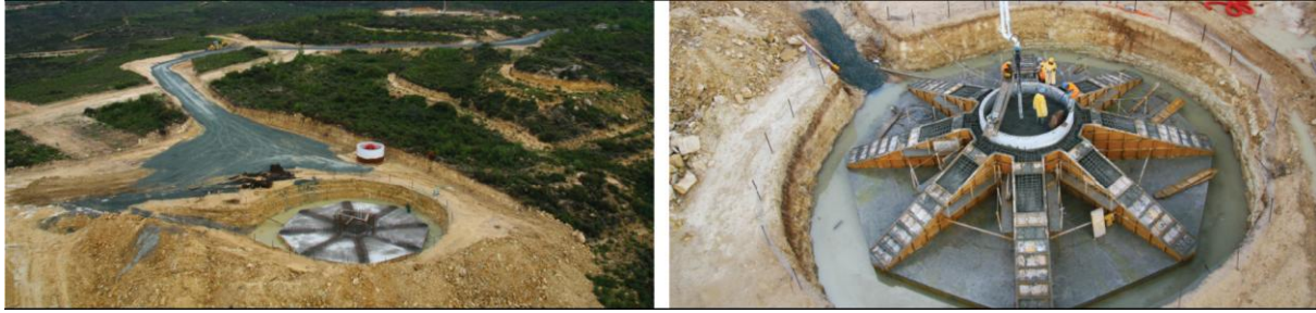
Photos from the construction of the first Wind Farm at Orites locality in the area of the villages of Pano Archimandrita, Kouklia and Alektora in the districts of Paphos and Limassol.
